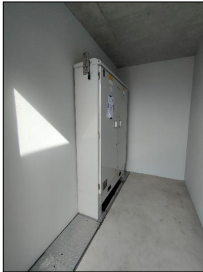
Figure 9 – Power supply unit.
