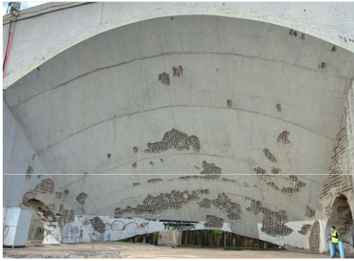
Figure 4 – Condition of Arcade 7 before intervention [1].
