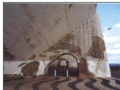
Figure 3 – Pre-existing damage in the columns [1].
