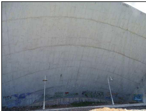
Figure 5 – Condition of Arcade 3 before intervention [1].
