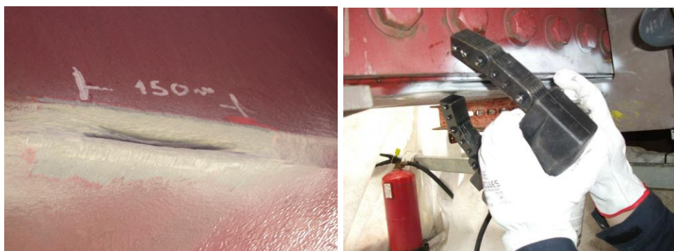
Fig. 4 A seam weld prepared for welding after preparation of surface. Fig. 5 Magnetic particle testing after welding.
