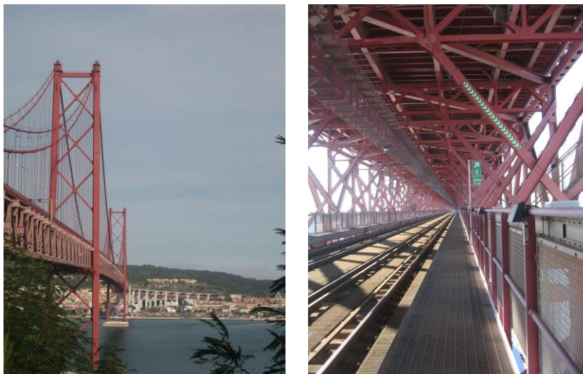
Fig. 1 South view of the Bridge over Tagus. Fig. 2 Inside view of the railway.
