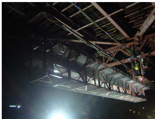
Fig. 8 Night installation works of the new modules of the central inspection walkway.
